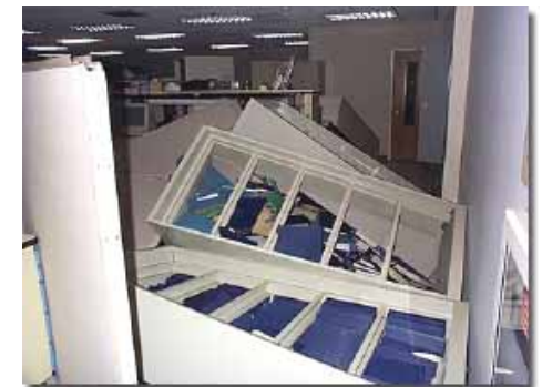
This example of non-structural damage is common after earthquakes of even moderate size - FEMA File Photo
