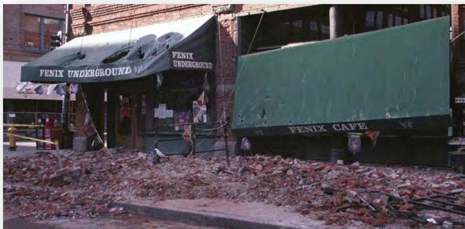
FEMA News Photo - This damage, from the 6.8M Nisqually Earthquake in 2001, could have been prevented or minimized had earthquake mitigation been employed. No one was hurt in this example, but building facilities and business operations were impacted
