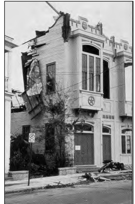
Historic site 12 Vanderhorst St. received damage during Hurricane Hugo. The site has since been restored.
